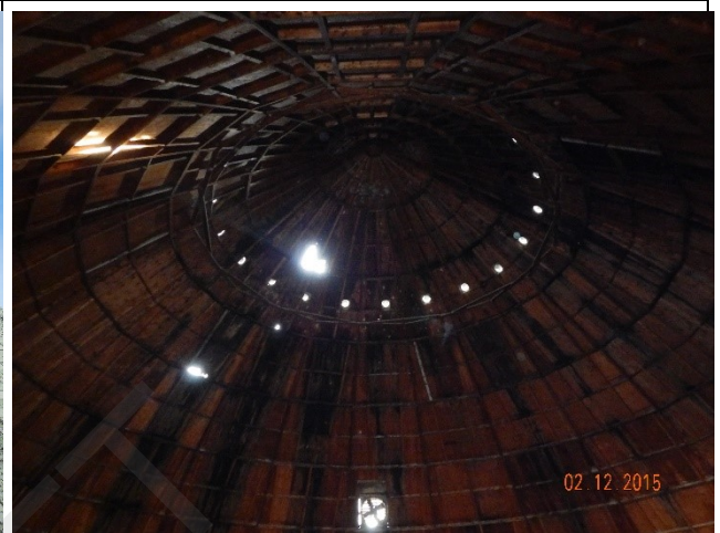
Damage inside of salt dome
