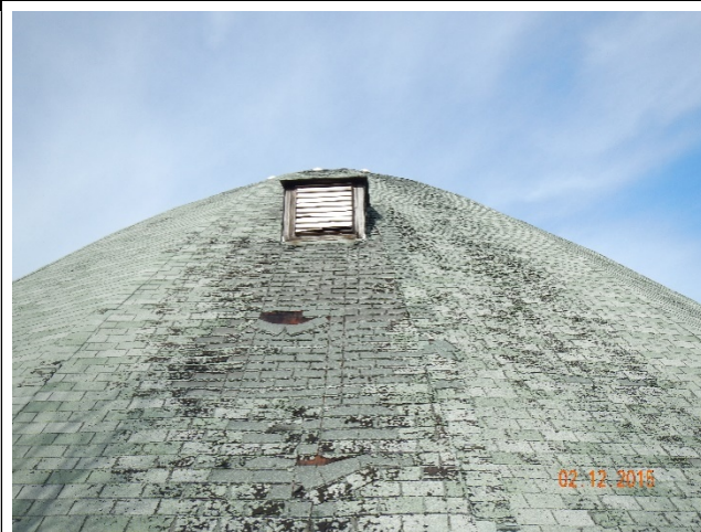
Salt dome shingle damage
