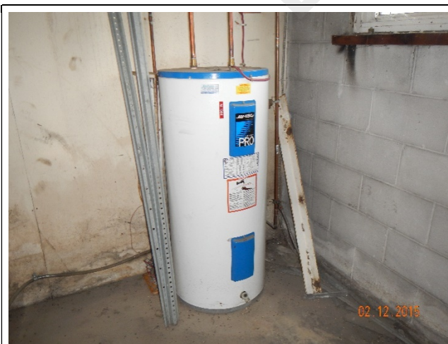
Electric hot water tank
