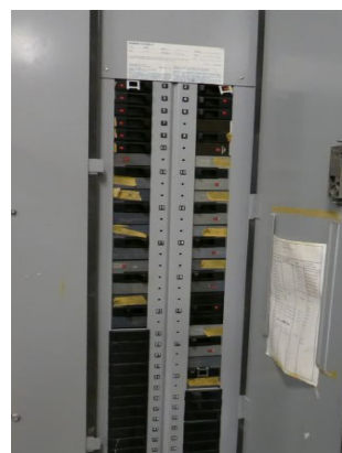
Figure 28 – Typical Distribution Panel
