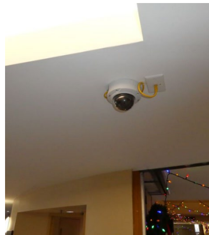
Figure 34– CCTV Camera in use on Main floor
