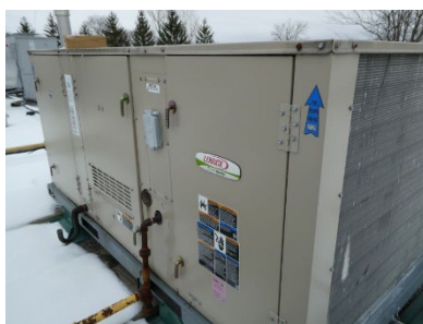
Figure 21 – Gas Fired Roof Top Unit
