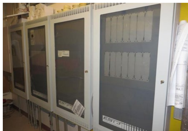
Figure 25- Fire Alarm Panel Typical
