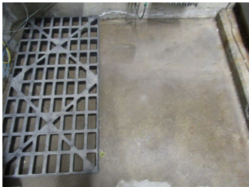
Figure 1- Foundation Leaking - Main Electrical Room Basement Level
