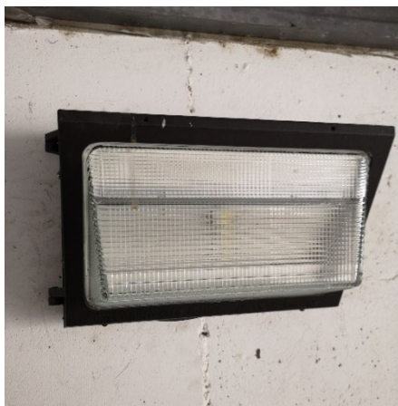
Figure 29 – Exterior LED Wall pack
