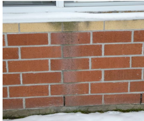
Figure 6 – Exterior Brick Effluence
