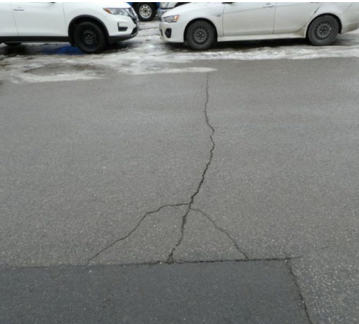
Figure 40 – Asphalt cracking- Northwest parking
