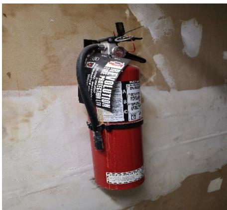
Figure 24 – Fire Extinguisher – Mechanical Room
