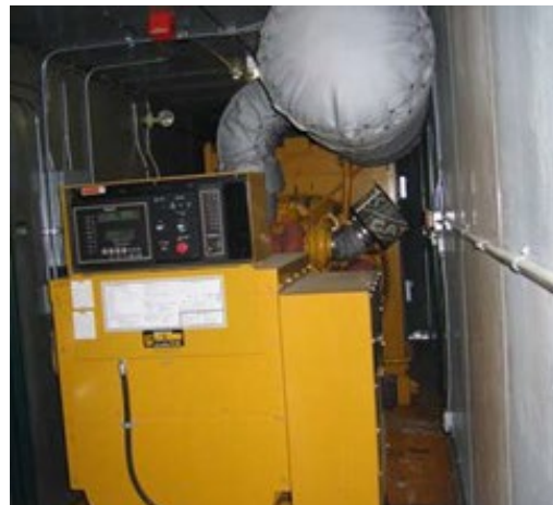
Figure 36 – 1000KVA Gas Generator
