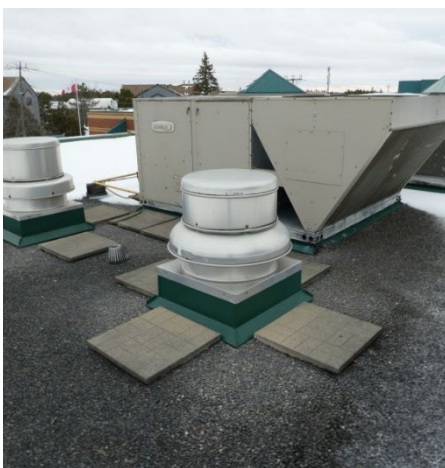
Figure 10 – Rooftop HVAC Units
