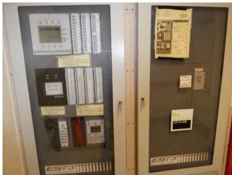
Figure 31 – FACP – Main floor Fire Fighters Entrance
