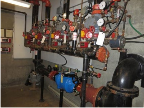
Figure 26- Main Sprinkler Incoming
