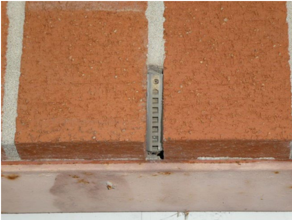
Figure 5 – Exterior brick expansion joints Deterioration
