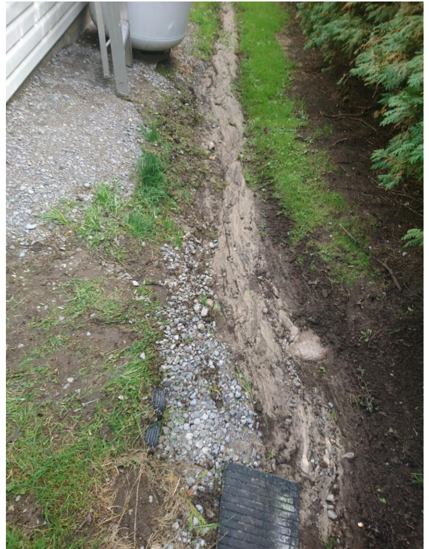
Summer Erosion after a typical rain storm
