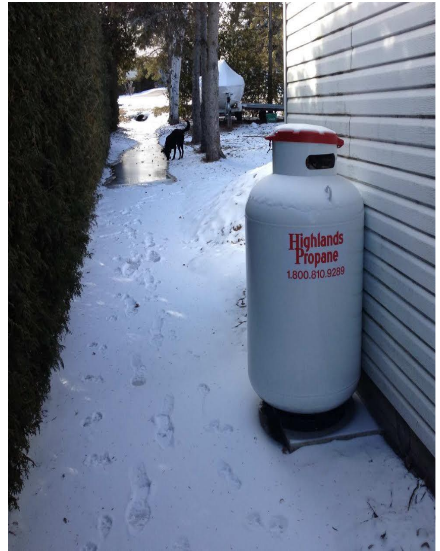
(The starting of the thaw) Refreezing over the small swale and eroding the hedges, trees, driveway and undermining the buildings foundation
