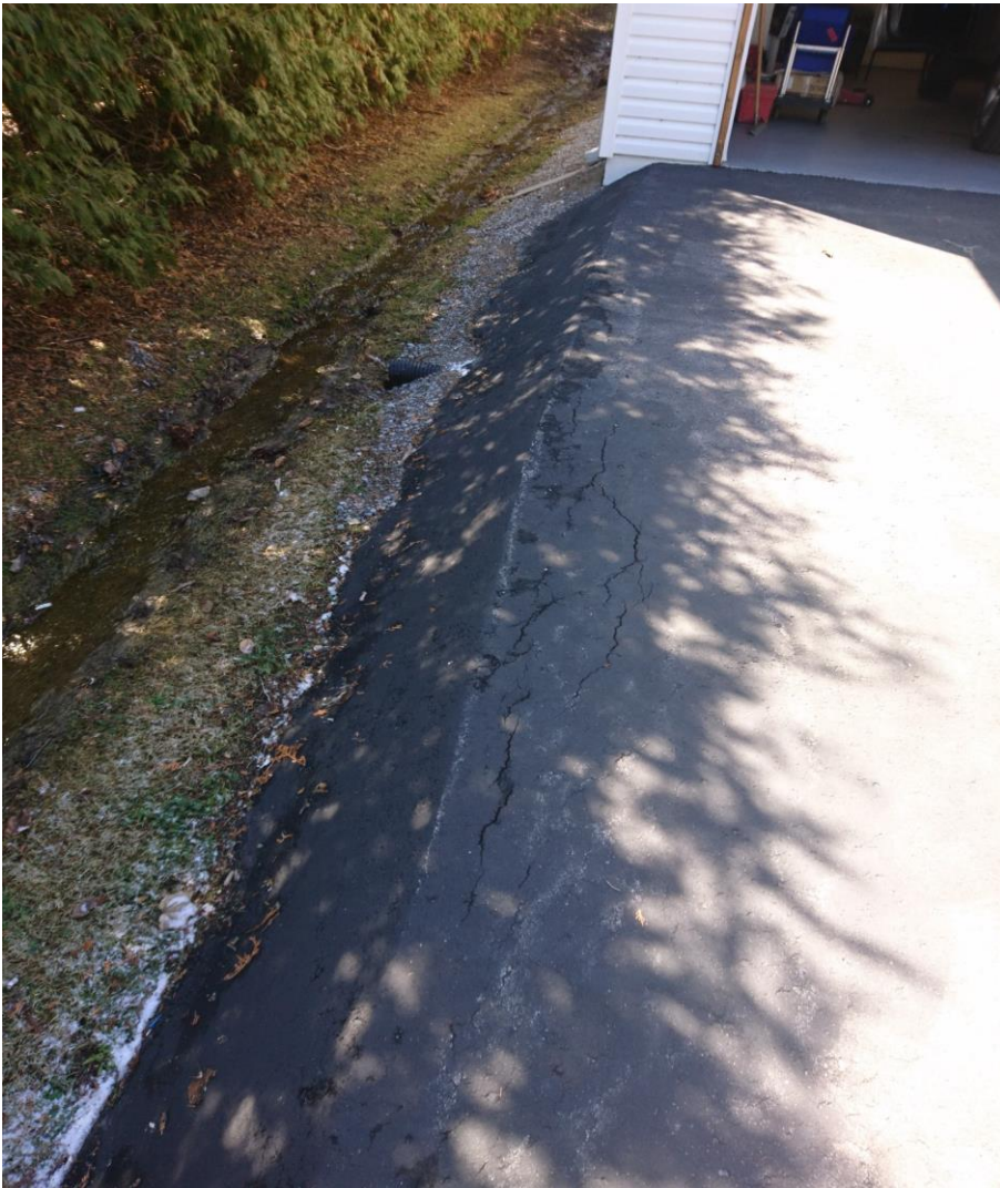
Erosion and splitting of driveway due to erosion and soft soil.
