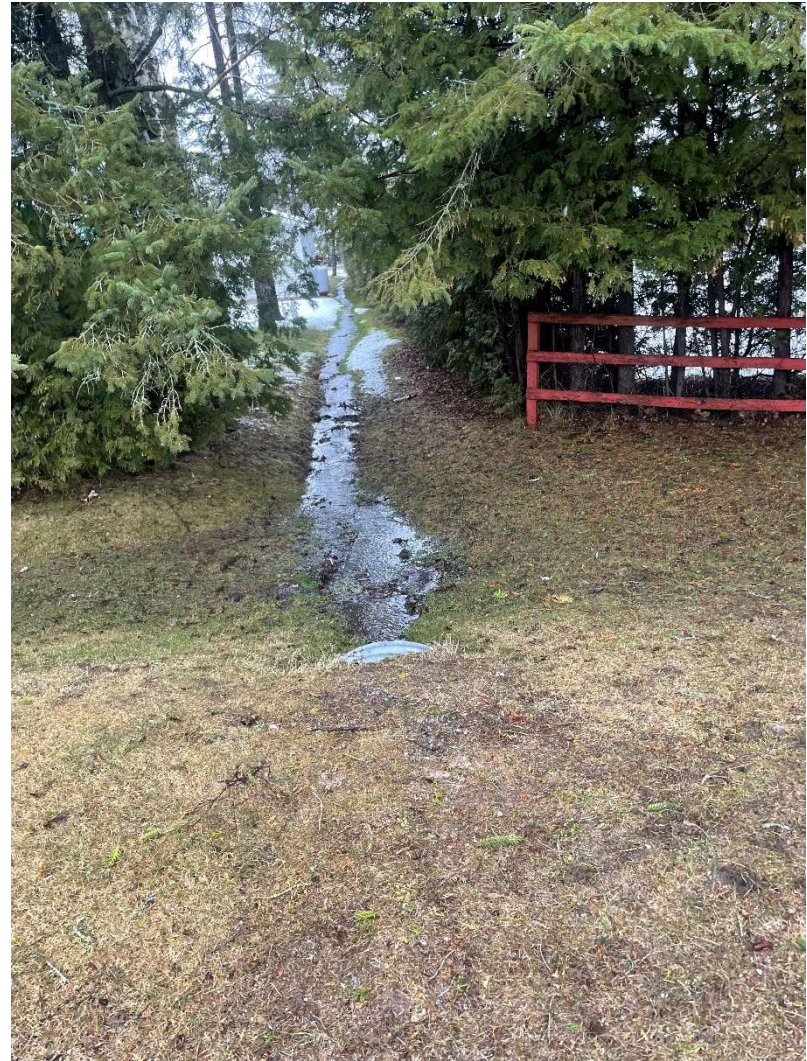
View south from Cameron Drive at existing drainage ditch at 149 Fenlon Drive
