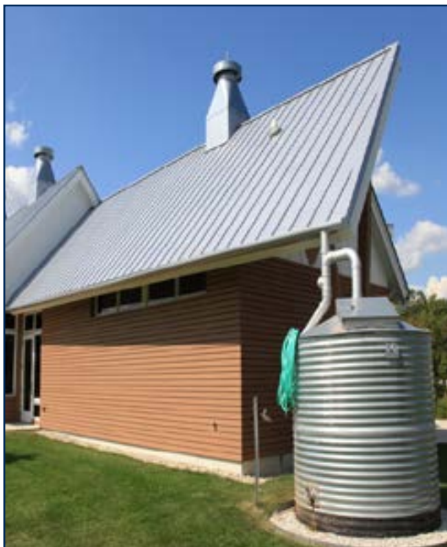
An example of a rainwater cistern. These are available in many shapes and sizes and may be above or below ground.
