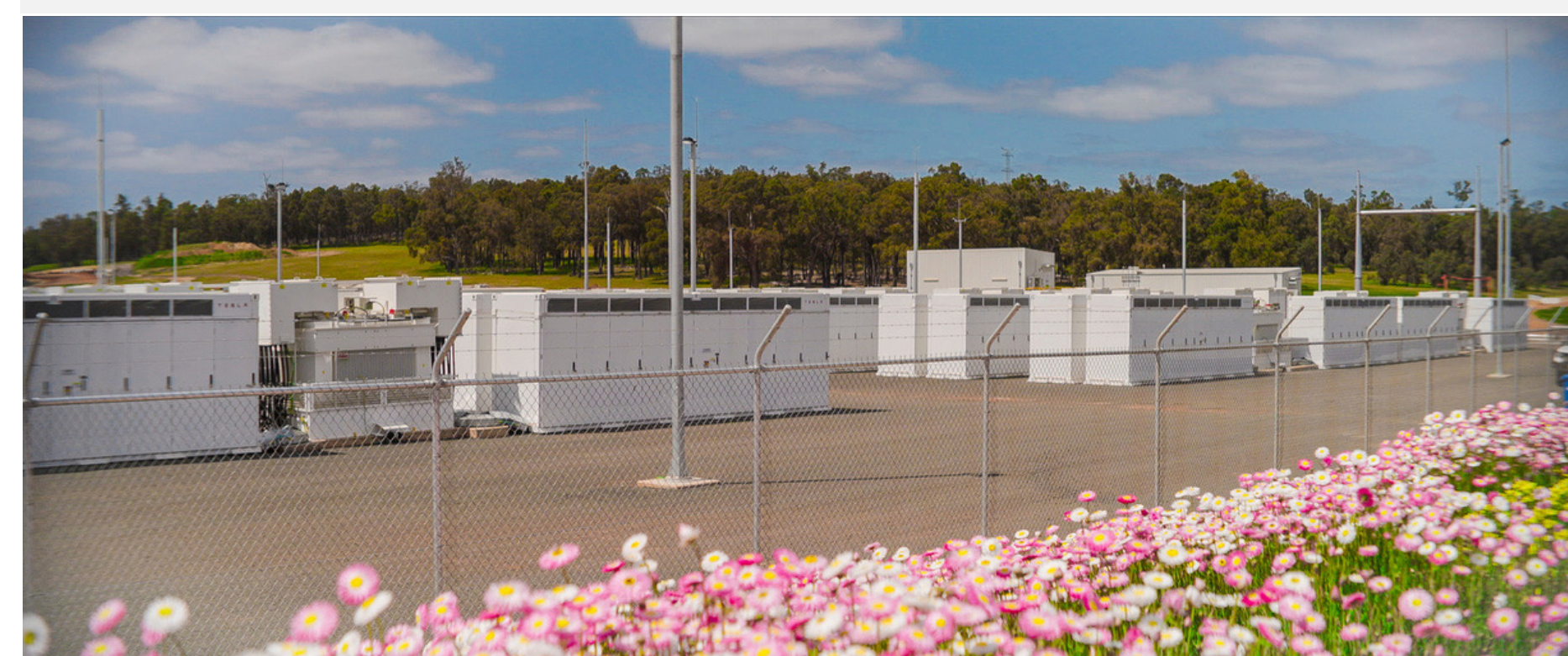
COLLIE BATTERY, AUSTRALIA (219 MW / 877 MWh)
