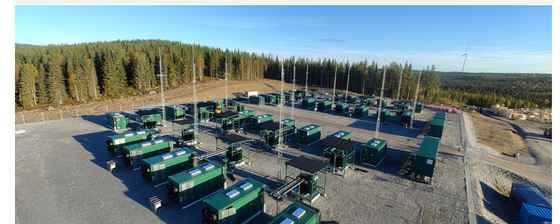
ISBILLEN POWER RESERVE, SWEDEN (93.9 MW / 93.9 MWh)
